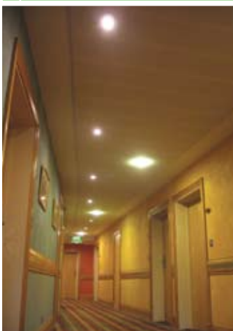
Corridor Office Surrey 5 watt "Antares" downlight- ers replacing 35 watt halogen downlighters
